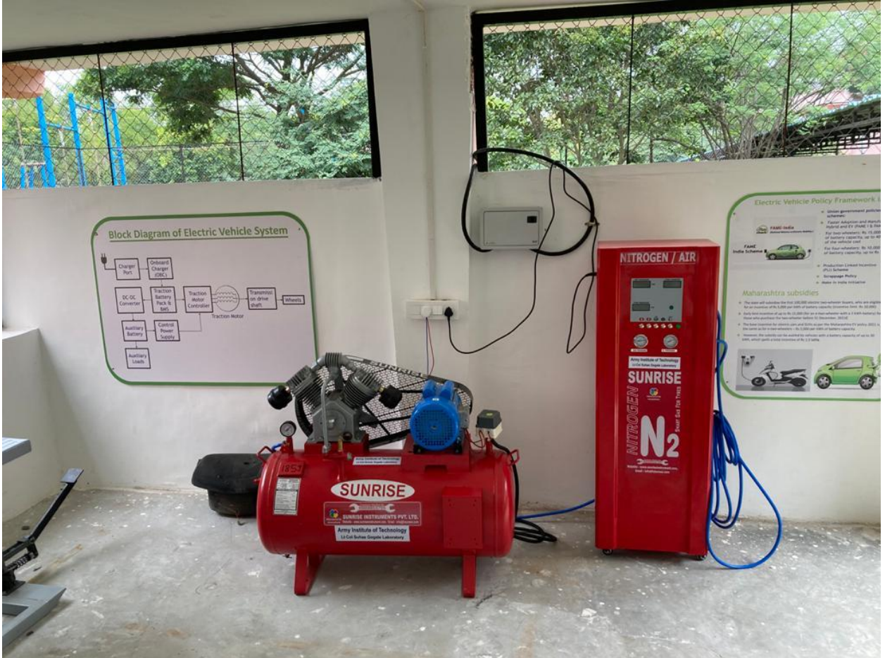
Nitrogen/air filling station
